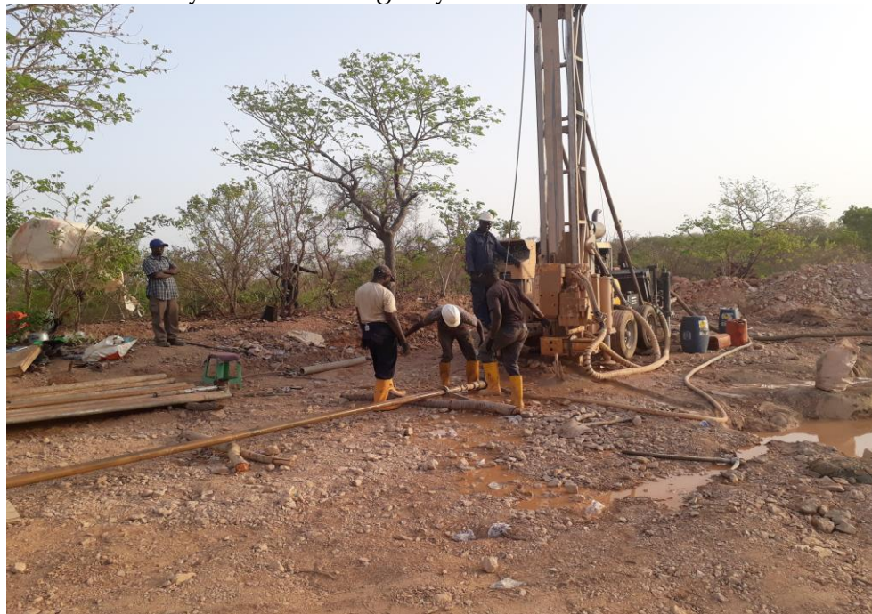
Angular Core Drilling Operation at Garin Auwal Gold Project, Fakai LGA, Kebbi State
